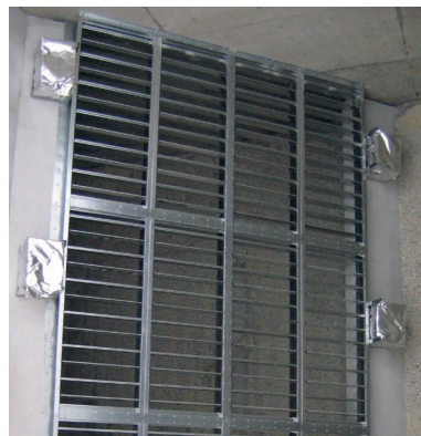
Multi-module of 6 MO-D dampers on a road tunnel application. The total section = 4300 x 6200 mm.
